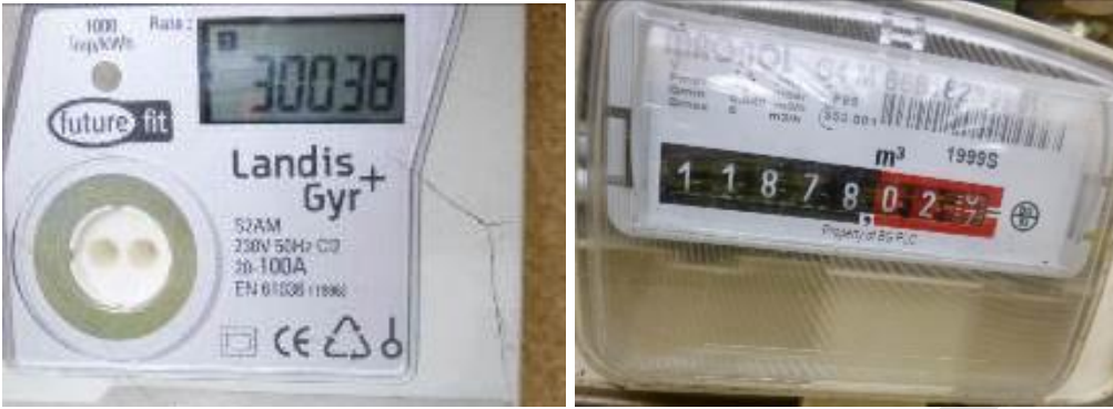
Electric and gas meter readings
